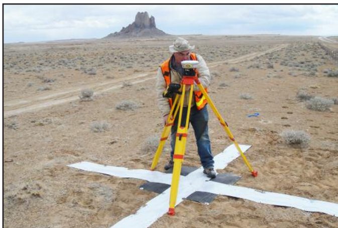
Survey work begins for the Navajo-Gallup Water Supply Project on the Navajo Nation. U.S. Bureau of Reclamation
