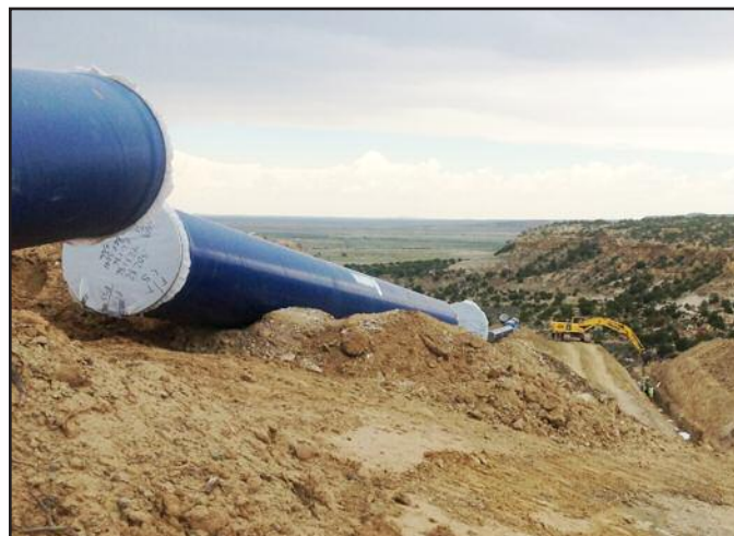
Pipes are laid for the Navajo-Gallup Water Supply Project Navajo Nation. Northwest New Mexico Council of Govts.
