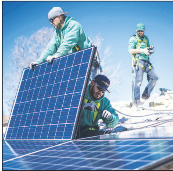
Workers secure rooftop solar panels in Albuquerque, New Mexico. A study estimates that 100,000 jobs will be created by 2050 if the state switches from fossil fuels to 100% renewable energy. Sergio Flores/Bloomberg via Getty Images
